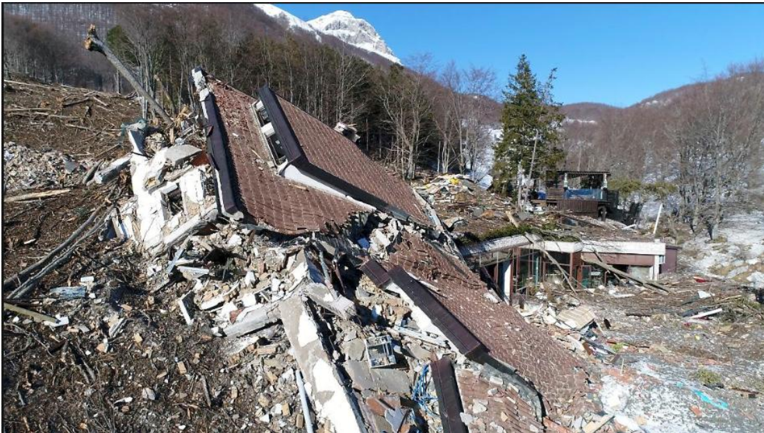
Figure 6.16: On January 18th, 2017, the Rigopiano Hotel was destroyed by a powerful avalanche. The force of the avalanche displaced the structure by at least 10 meters. Notably, the building appears detached from its foundation and is visibly tilting backward.
